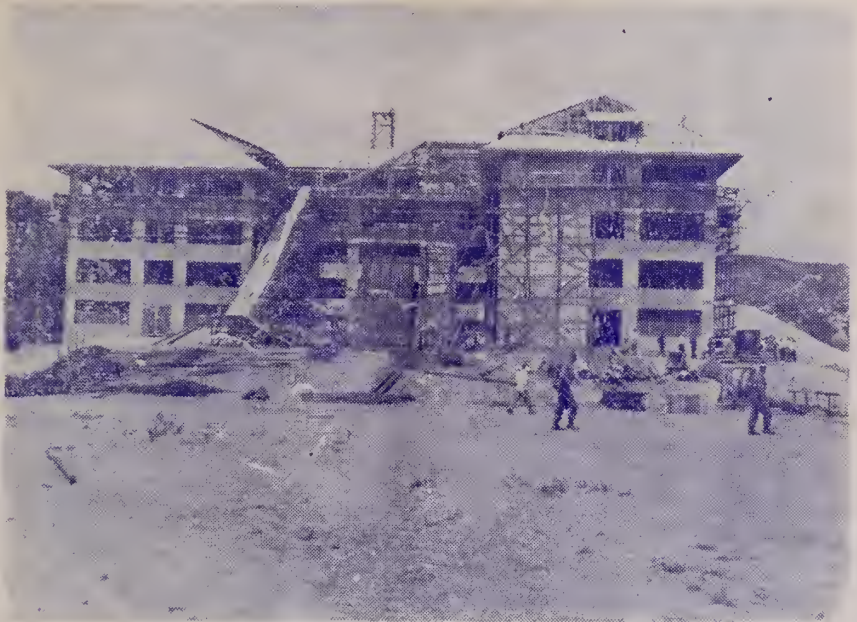
8th U.S. Army Memorial Chest Surgery Hospital Under Construction with the Assistance of 8th U.S. Army in Korea
